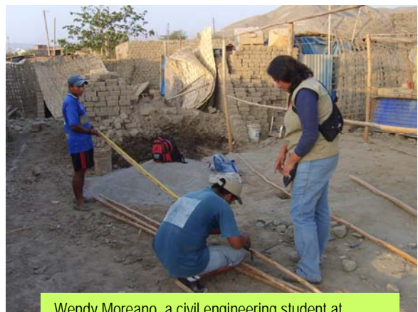
Wendy Moreano, a civil engineering student at Universidad San Luis Gonzaga, provides guidance on how to construct transitional shelters.
